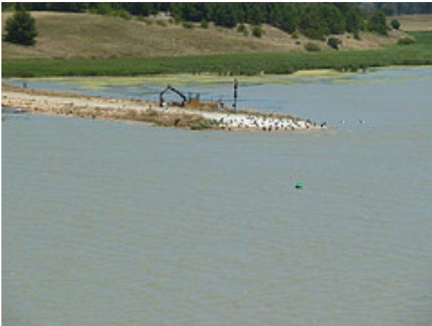
Clayton Bay regulator – river still partially blocked.
