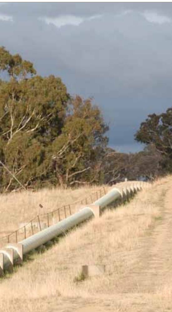
Water pipes from the Cotter River to supply Canberra, Australian Capital Territory
