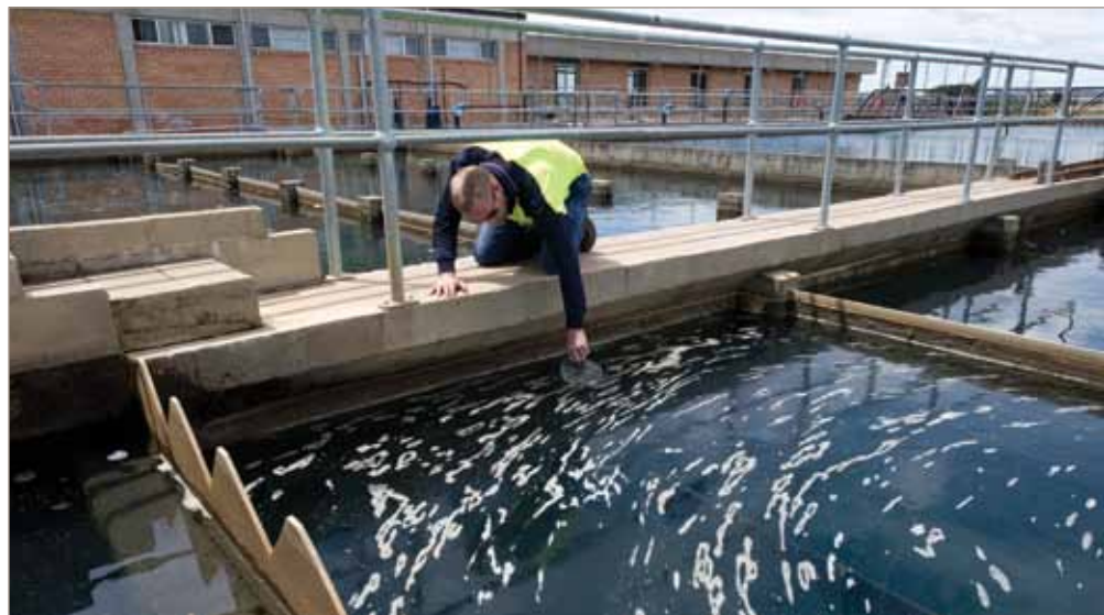
Testing the water of sedimentation and flocculation tanks at a water treatment plant at Bathurst, New South Wales
