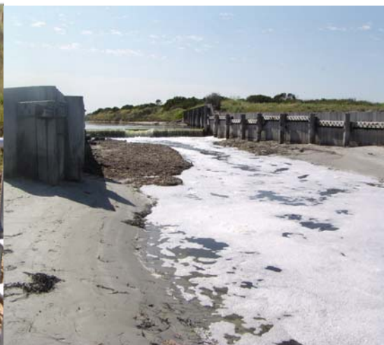
Drain discharge –Southern Ocean - Kingston South East (SA) Drains (photo L Burge)
